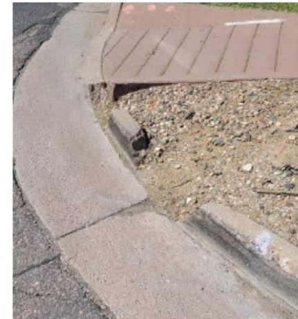
Curb head completely spalled
