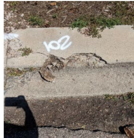
Surface spalling of curb face
