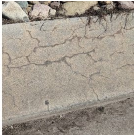
Minor surface cracking
