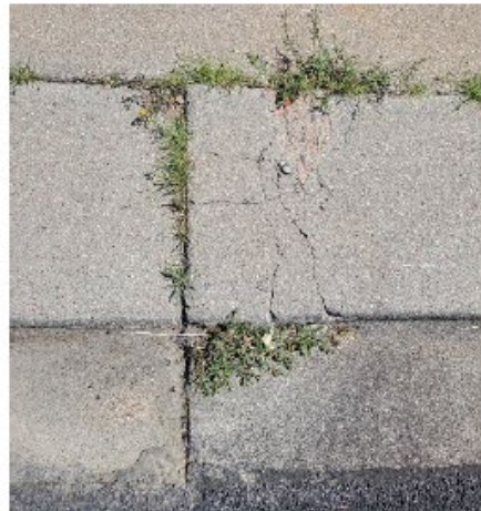
Mild surface cracking with some spalling
